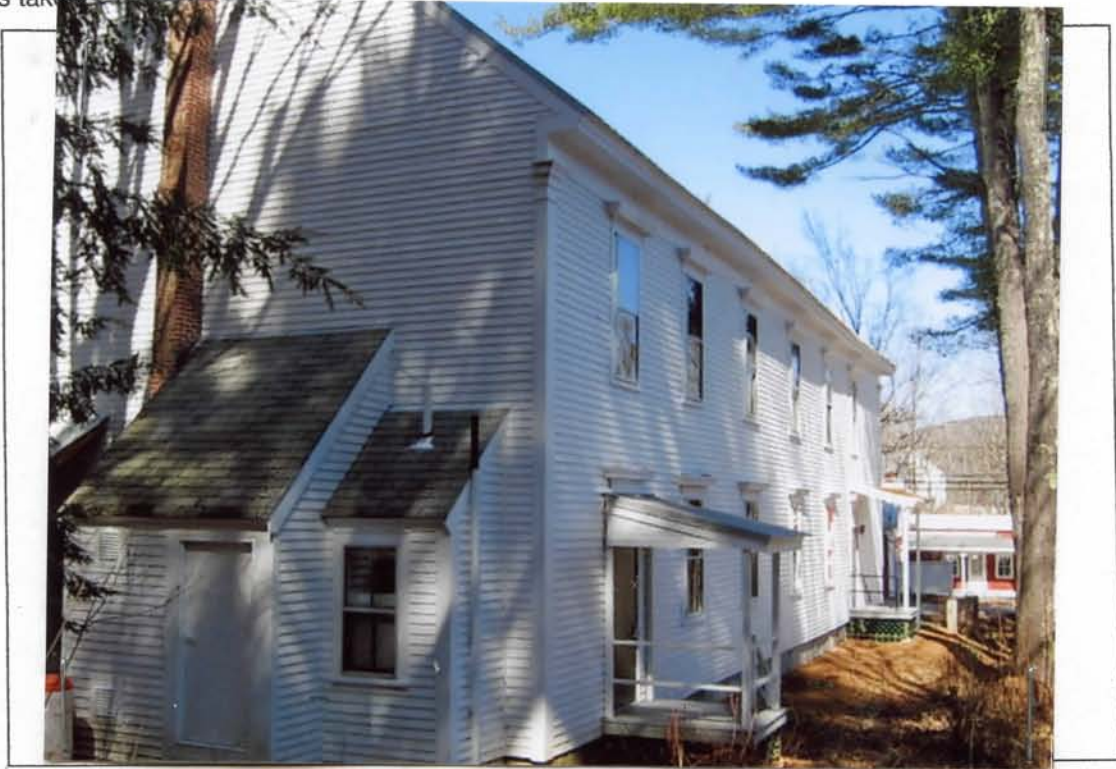
Photo # 6 Description: South side entrance / exits Roll and Frame # OR Digital file name: Town Hall exterior 3082 Direction: South
