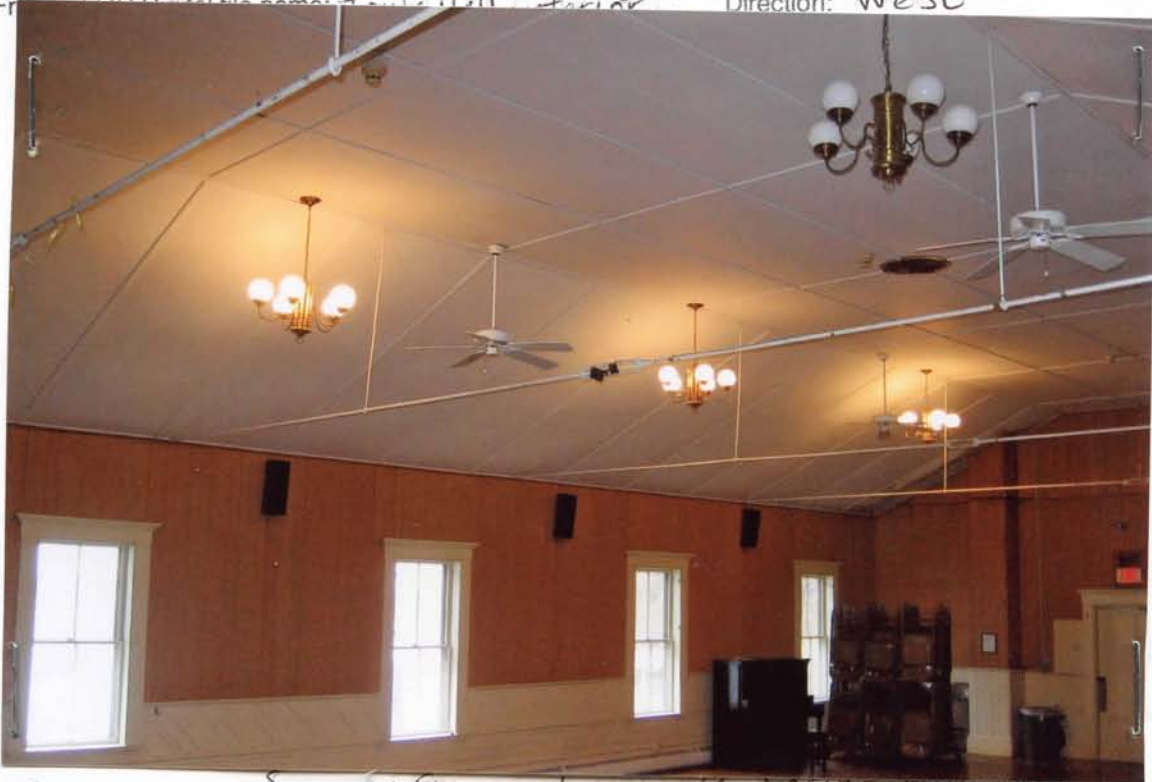
Photo # 17 Description: Second floor ceiling, north facing windows Roll and Frame # OR Digital file name: Direction: northeast
